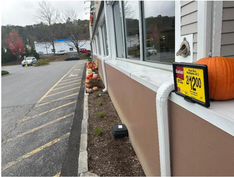
Figure 28 Flood wall with flushing, rerouted downpipes, and vents.
