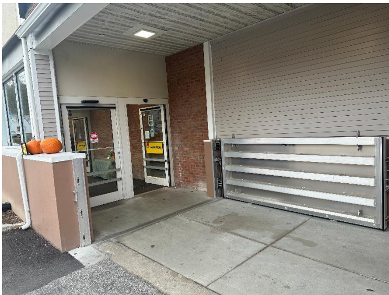
Figure 29 Flood gate at the main entrance, must be manually closed and locked during deployment
