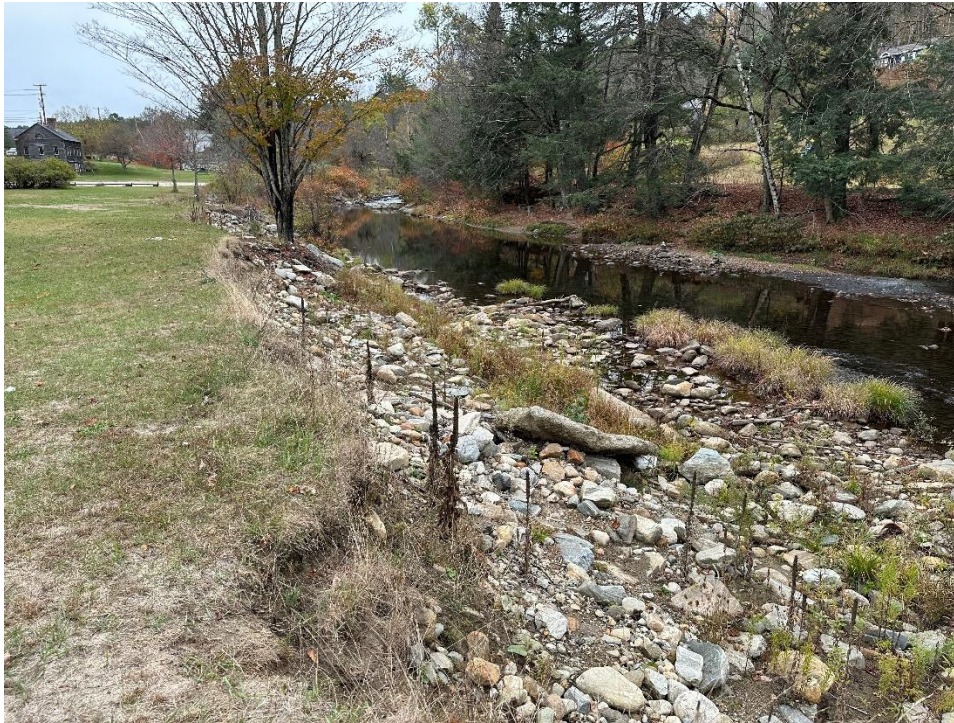
Figure 3 Eroded right embankment of the West River displaying loose sandy soil with a high rock content.
